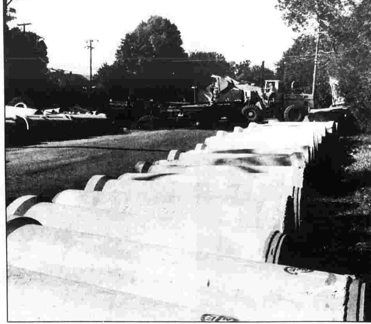
WAITING IN LINE — Sewer pipes are lined up, ready to be buried on Oak Grove Street in Manchester by Central Paving Inc. of South Windsor.
